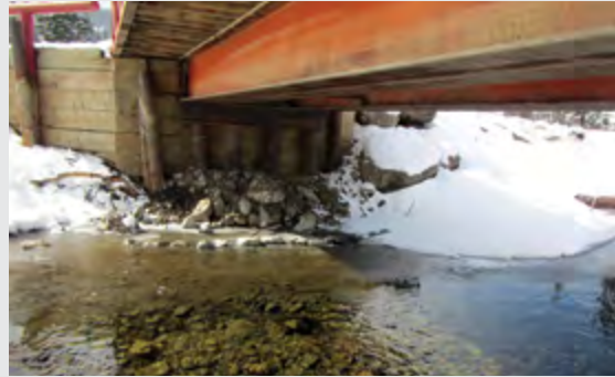
Sites showing unsuitable fill material used for stabilization, impacting the habitat and spawning areas for Westslope Cutthroat Trout
